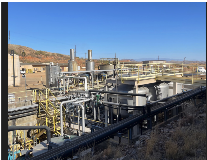
Figure 17-12: JCM Tank Farm
