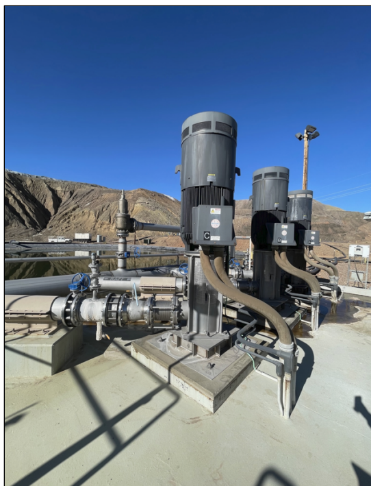
Figure 17-7: Raffinate Pumps at JCM
