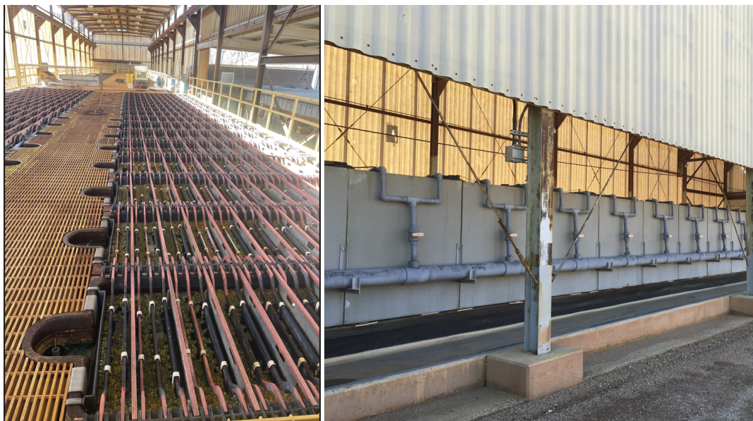
Figure 17-11: JCM EW Tankhouse Interior and Exterior
